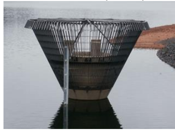
© Photo EDF Sambarino Spillway morning glory
