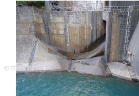
© Photo EDF right bank bottom outlet downstream deflector
