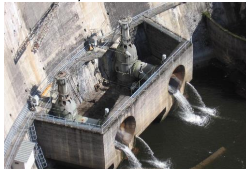
© Photo Coyne et Bellier Bottom outlets
