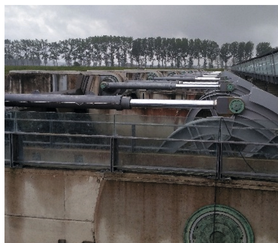
Figure 8.20 – Actuators, arms and sluice actuators, at high tide / © BRli
