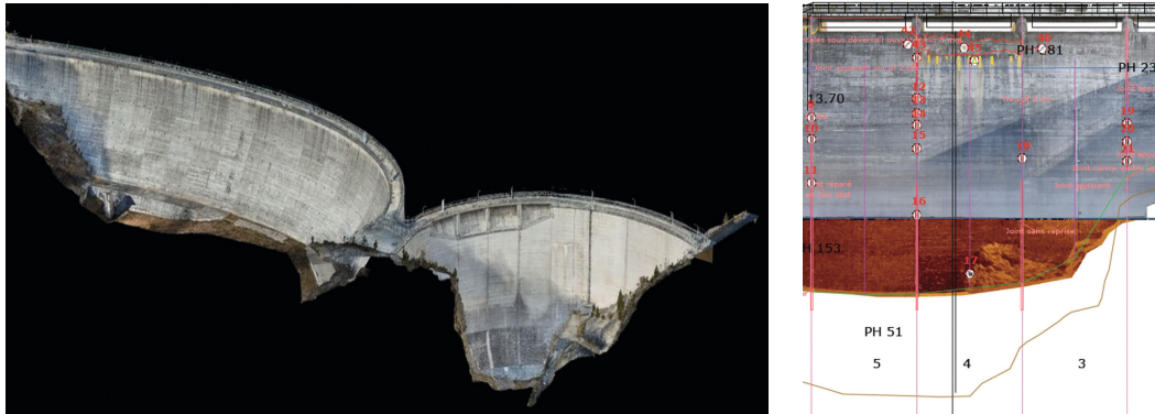
Figures 11.13 et 11.14 – Exploitation of UAV shots: on the left 3D model and on the right plotting of inspection results on 2D orthophotos / © EDF
