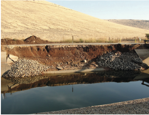
Figure 7.10 – Friant Kern Canal (USA, 2012) – Typical failure of the concrete protection slab of the embankment due to the presence of expansive soils / @ Lhoist
