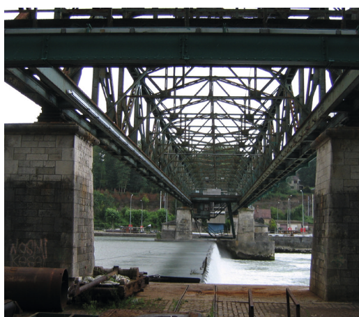
Figure 8.11 – Old barrage in operation since 1928, fitted with Aubert flashboards / © Artelia
