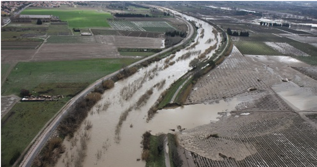
Figure 9.8 – Breach on the Agly levees in 1999 / © DREAL Occitanie
